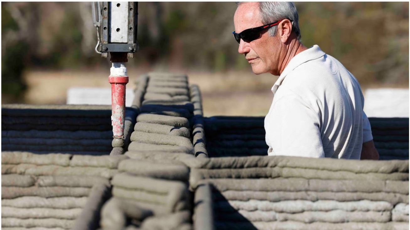
Craig Pettit, president of MRB Robotics, monitors a 3D printer as it adds a layer of concrete to a future self-storage facility in Payne Springs. (Shafkat Anowar / Staff Photographer)
