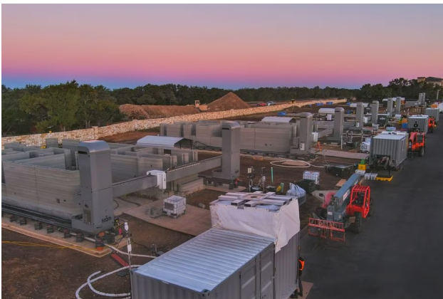
A fleet of 3D printers construct the walls of new homes in the Wolf Ranch residential community in Georgetown. (Icon)
